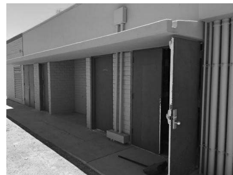
NORTH DOORS - TO BE REPLACED
