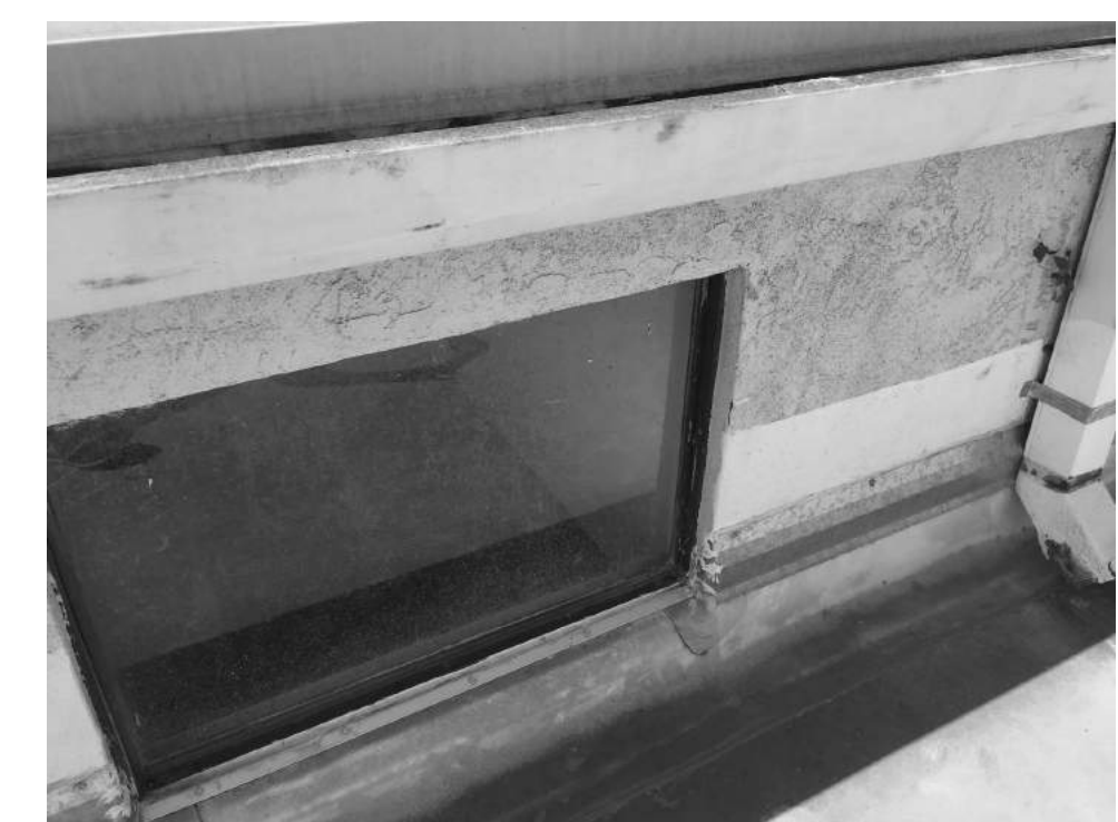
EXISTING CLERESTORY WINDOW TO BE REPLACED
