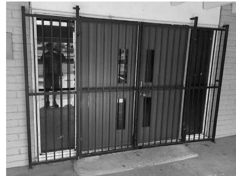
ENTRY DOORS WITH SECURITY
