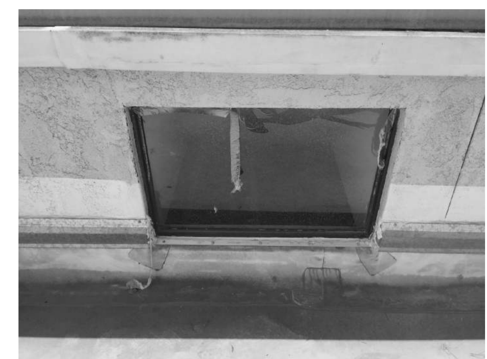
EXISTING CLERESTORY WINDOW TO BE REPLACED
