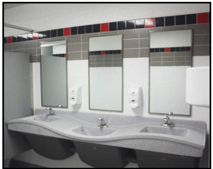
The Gymnasium area rest rooms after having been re-modeled to very modern standards.
