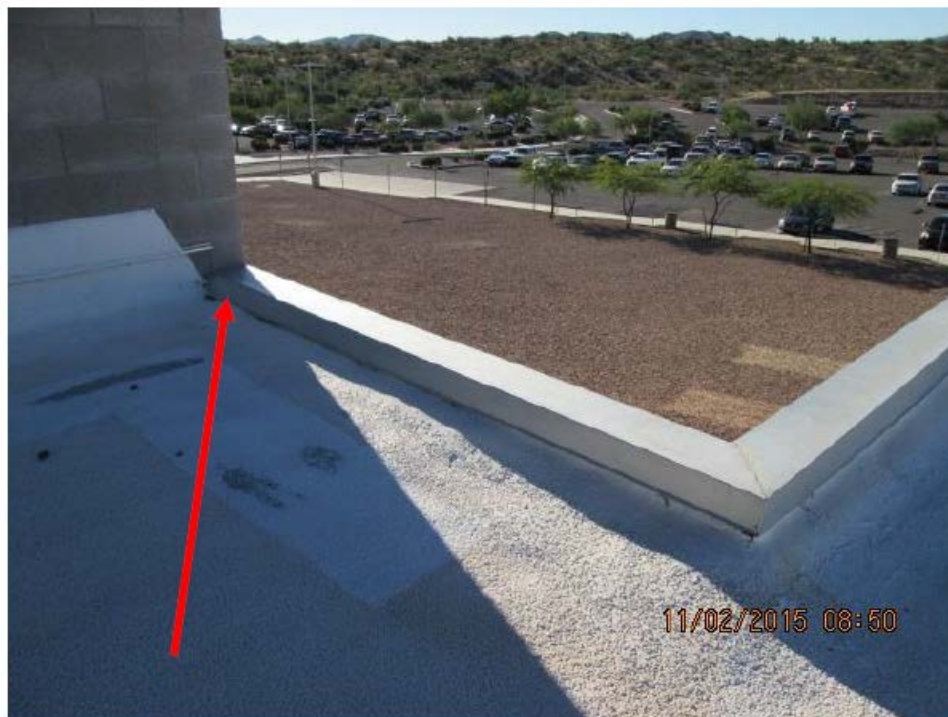
Typical coping condition that needs to be modified on Roof Section #1
